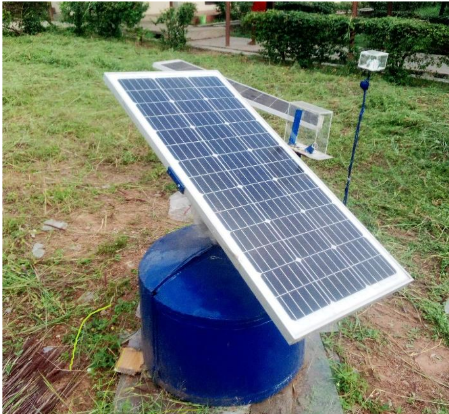
Fig. 3. Dual axis solar power generating system
